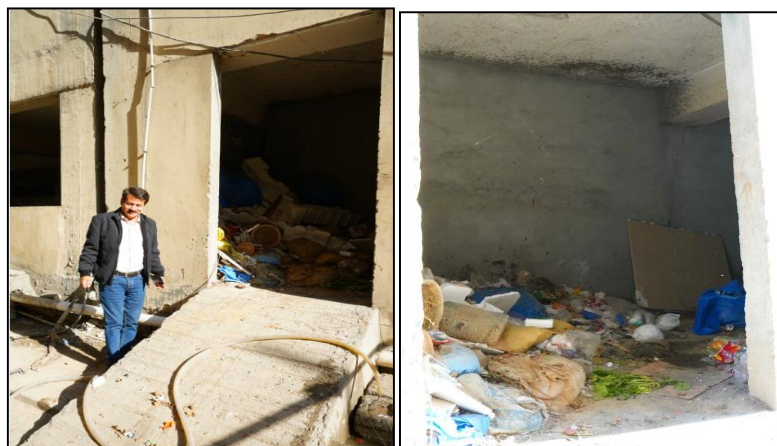
Figure 11 Removed waste temporary dumping site next to parking
