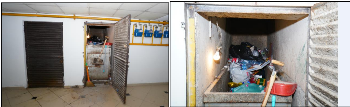
Figure 09 Open garbage chute site with access door opened for visit & dumped waste inside
