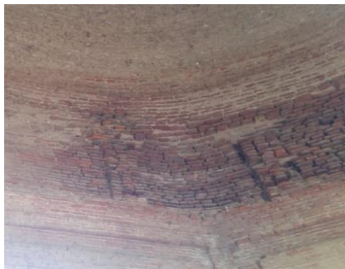
Figure 21 Damages in Internal side of Dome
