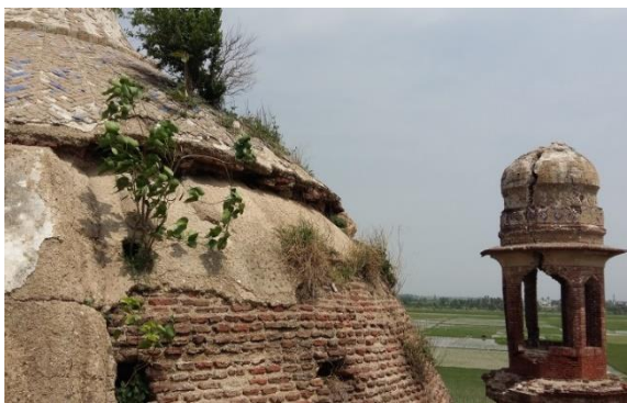
Figure 16: Structural Cracks in Copula of Minaret
