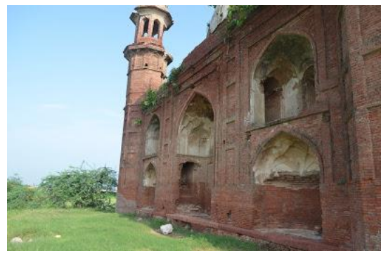
Figure 17: seepage of rain water
