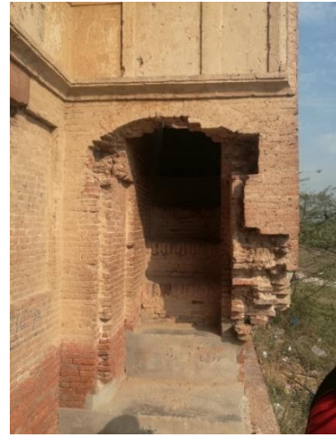
Figure 15: Structural damages due lack of maintenance
